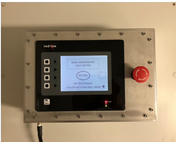
Figure 6.7. The "Reset" screen on the deck service box.
